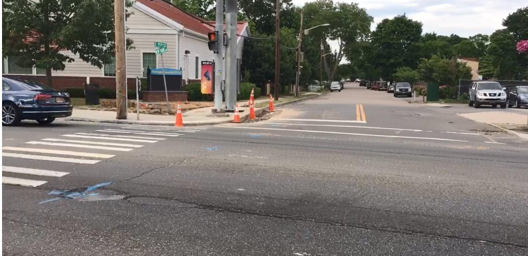
Construction observed blocking the sidewalk and crosswalk on the corner of E. 15 th Street and New York Avenue.
